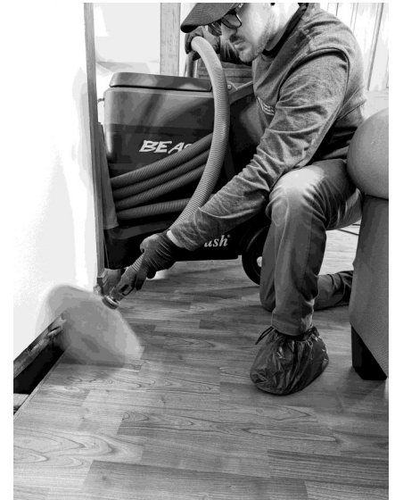
Above, VHP tech Rob Parker prepares to clean an air duct register using our Roto-Brush duct cleaning equipment..
