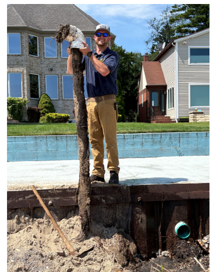
Marvin had to dig up and replace the line to get rid of this root mass.
