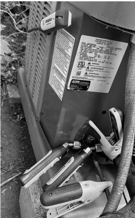
Here is a condenser with five mQ probes attached to measure the suction line & liquid line pressures and temperatures and also the discharge air temp.
